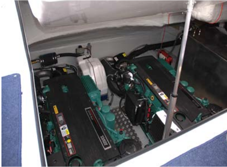
Spotless installation in the engine room is a testament to German engineering
